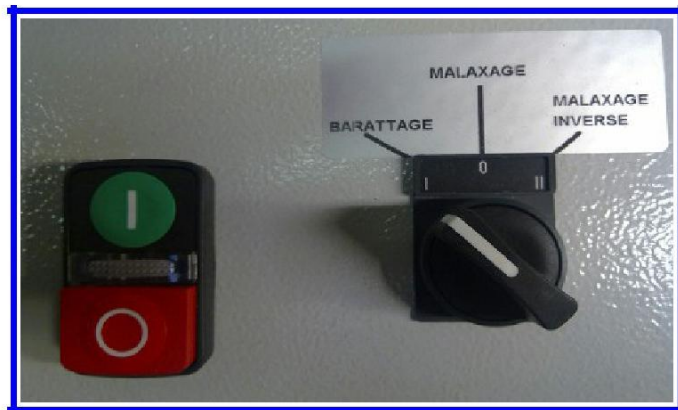
Command board Start/Stop push buttons with light on. Churning /kneading selector.
